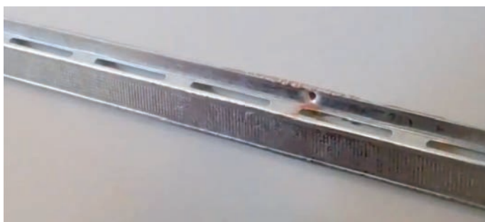
Figure 4: Still image from a how-to video 5 that shows RC being installed incorrectly
